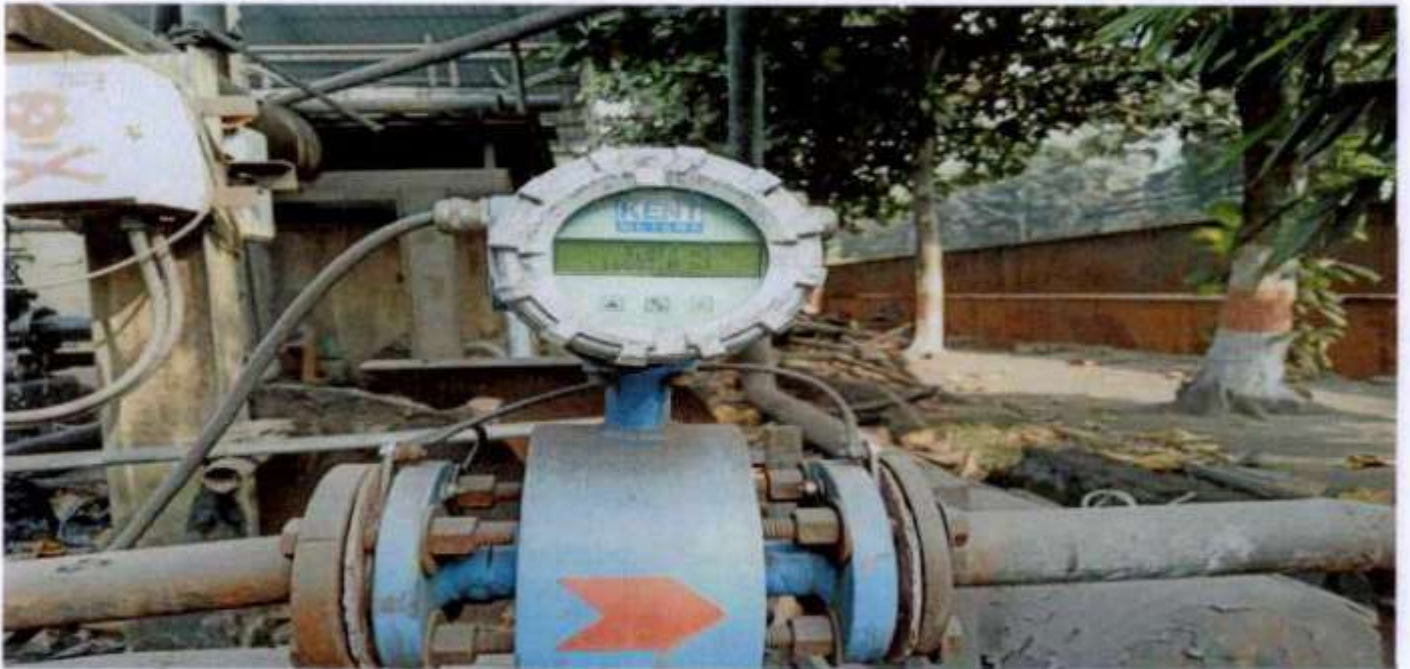
Bore with Digital Water Meter near Cooling Tower
