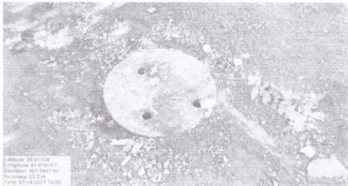
Structure 02 Recharge well 1 m dia 2 m depth
