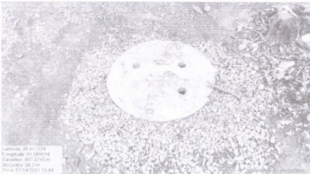
Structure 10 Recharge well 1 m dia 2 m depth
