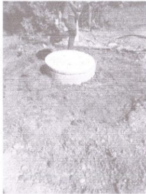
Structure 13 Recharge well 1 m dia 2 m depth
