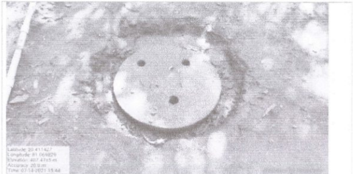
Structure 01 Recharge well 1 m dia 2 m depth
