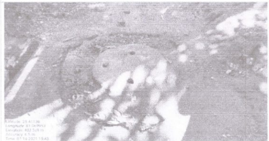
Structure 04 Recharge well 1 m dia 2 m depth
