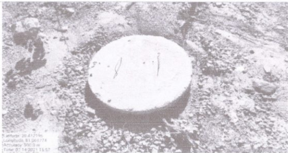
Structure 08 Recharge well 1 m dia 2 m depth
