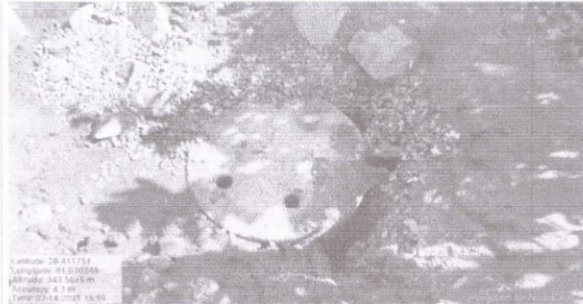
Structure 03 Recharge well 1 m dia 2 m depth
