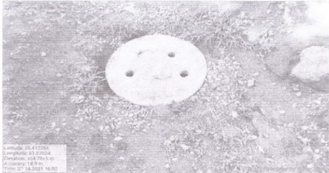
Structure 07 Recharge well 1 m dia 2 m depth
